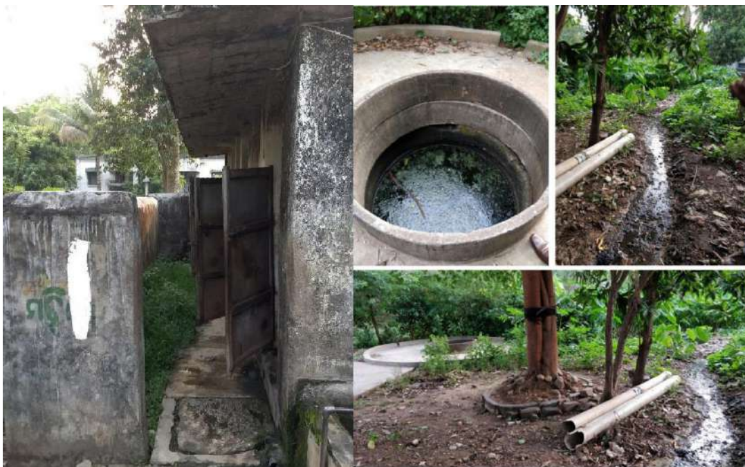
Figure 1: Water and Sanitation Condition Before Intervention (Toilet Infrastructure and open well)
