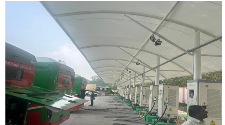
Charging Stations – Telangana
