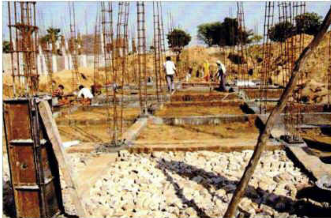
Actual site photograph of affordable housing project in Jaipur Development Authority region
