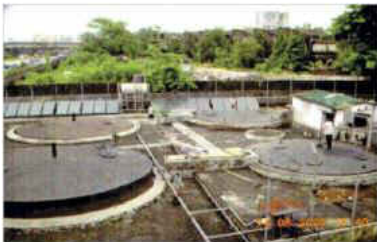
Bio Methanisation Plant
