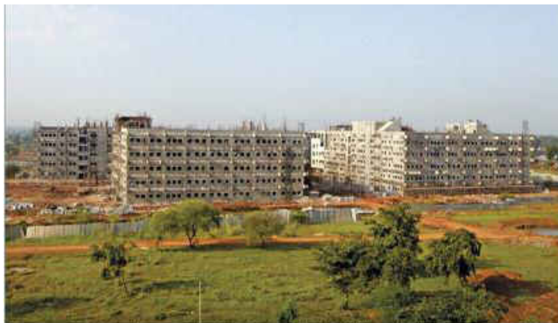
Capitol Complex comprising of the Secretariat, H.O.D. Building and Allied Facilities in Naya Raipur (nearing completion)
