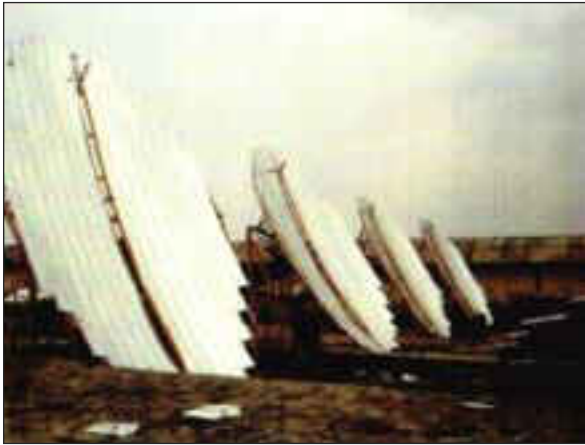
Solar Paraboloids as part of Air Conditioning System
