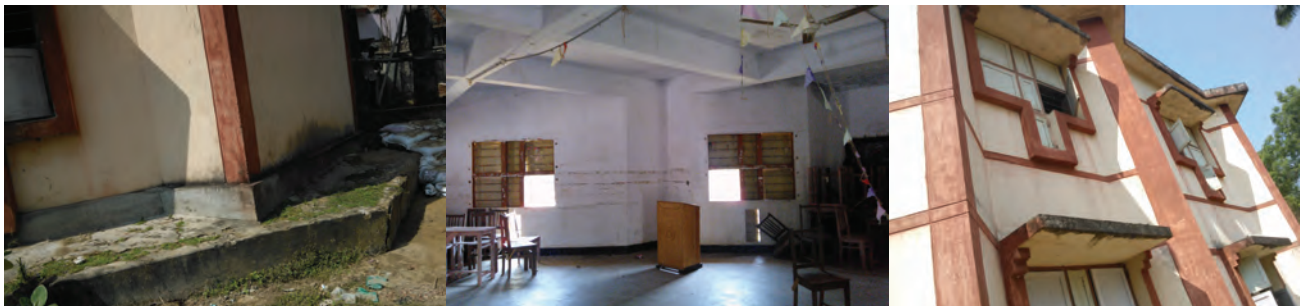
Figure 12: Lack of cleanliness, poor condition of plinth protection, Hall being used for storage, window shutters missing
