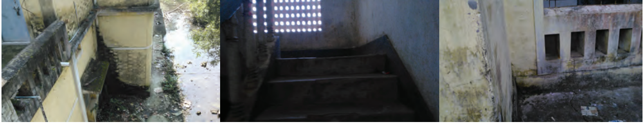
Figure 9 : Water logging/ lack of cleanliness, poor condition of staircase & plinth protection
